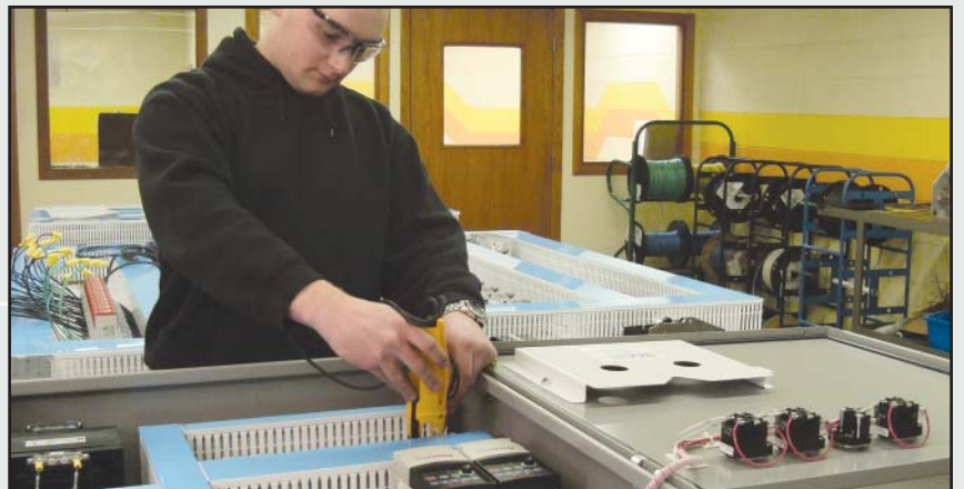
Electrical panel testing in Nercon's U.L. compliant panel shop.
