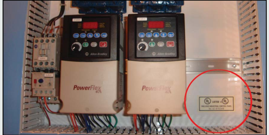
U.L. sticker is shown inside an electrical panel.
