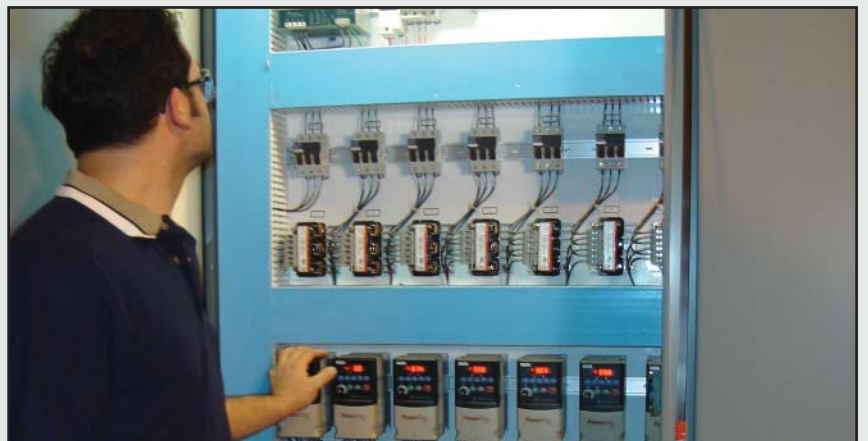
Electrical controls manager verifies panel operation.
