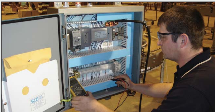
Nercon's controls technicians set up jobs in-house and travel to the customer site for start-up.
