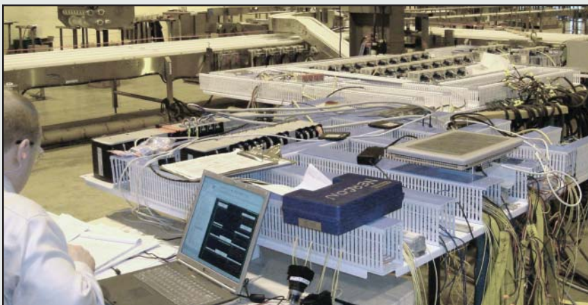
Nercon controls expert makes adjustments to the controls software during F.A.T.
