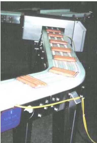
This conveyor system is integrated with a metal detector.
