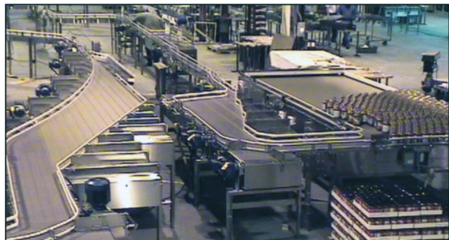
This system used expanded and optimized electrical controls to integrate all thermal controls and the high speed sauce line. The line was fully automated and menu driven with multiple HMI's.
